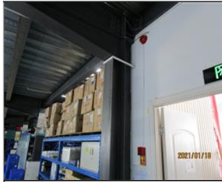
Photo of fire safety equipment Fire alarm.JPG
