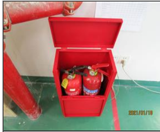
Photo of fire safety equipment Fire extinguishers.JPG
