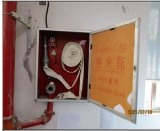
Photo of fire safety equipment Fire hydrant.JPG
